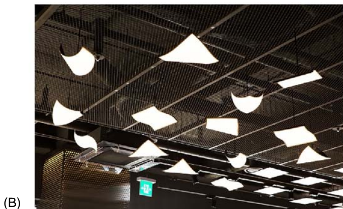
FIG. 5 (A) Comparison between LED and OLED lighting. (B) Flexible and rigid LG OLED light panels installed in Baskin Robbins commercial center (Seoul). Panel A: Reproduced from OLED Light, (2014). http://www.lgdisplay.com/eng/product/oled_light.jsp (Accessed 22 November 2020), © 2014 LG Display Co. Ltd; Panel B: Reproduced from Flexible and Rigid LG OLED Light Panels Installed in Baskin Robbins Brown Store, (2021). https://www.linkedin.com/pulse/flexible-rigid-lg-oled-light-panels-installed-baskin-robbins-chung (Accessed 22 November 2020), © 2017 LG Display Co. Ltd.
